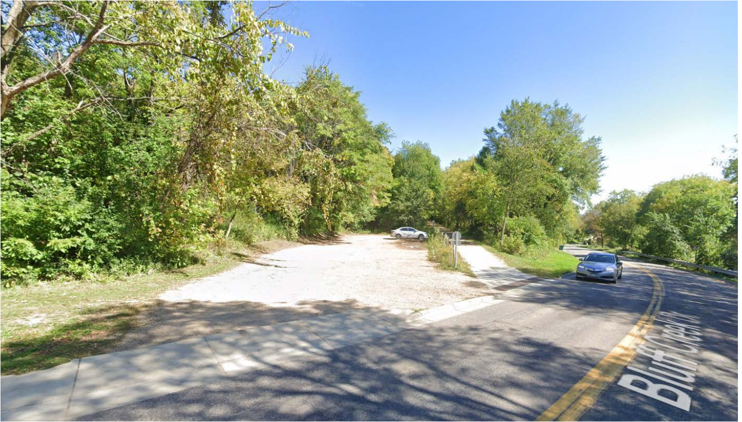
Unpaved parking lot, inaccessible surfacing, and lack of signage at Bluff Creek Drive (looking east)
