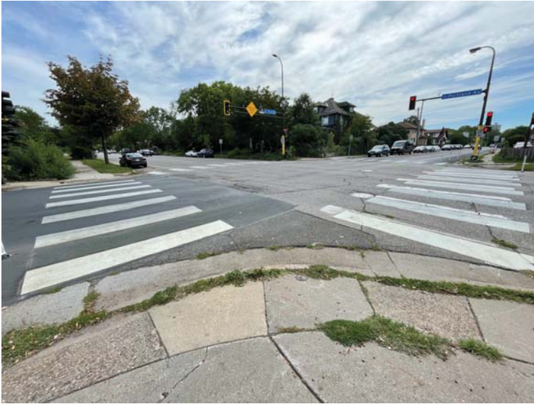
The intersection of Portland Ave (CSAH 35) and E 31st St contains non-compliant pedestrian ramps, similar to many intersections along the corridor.
