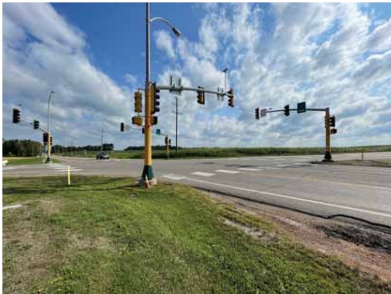
View of intersection at CR 116 (Fletcher Ln) and CSAH 10. The photo above shows that this intersection lacks sufficient ADA compliant pedestrian ramps for people walking and rolling.
