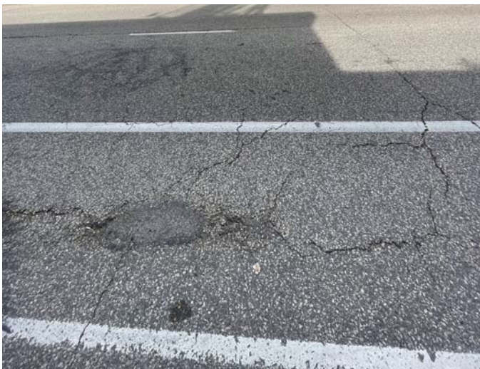
Pavement infrastructure is cracked and requires repairs.
