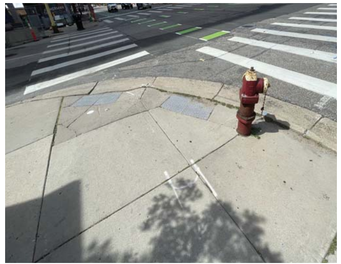
Many pedestrian ramps along the corridor are not compliant with current ADA standards such as those within the photo above at Washington Ave (CSAH 152) and Portland Ave (CSAH 35).
