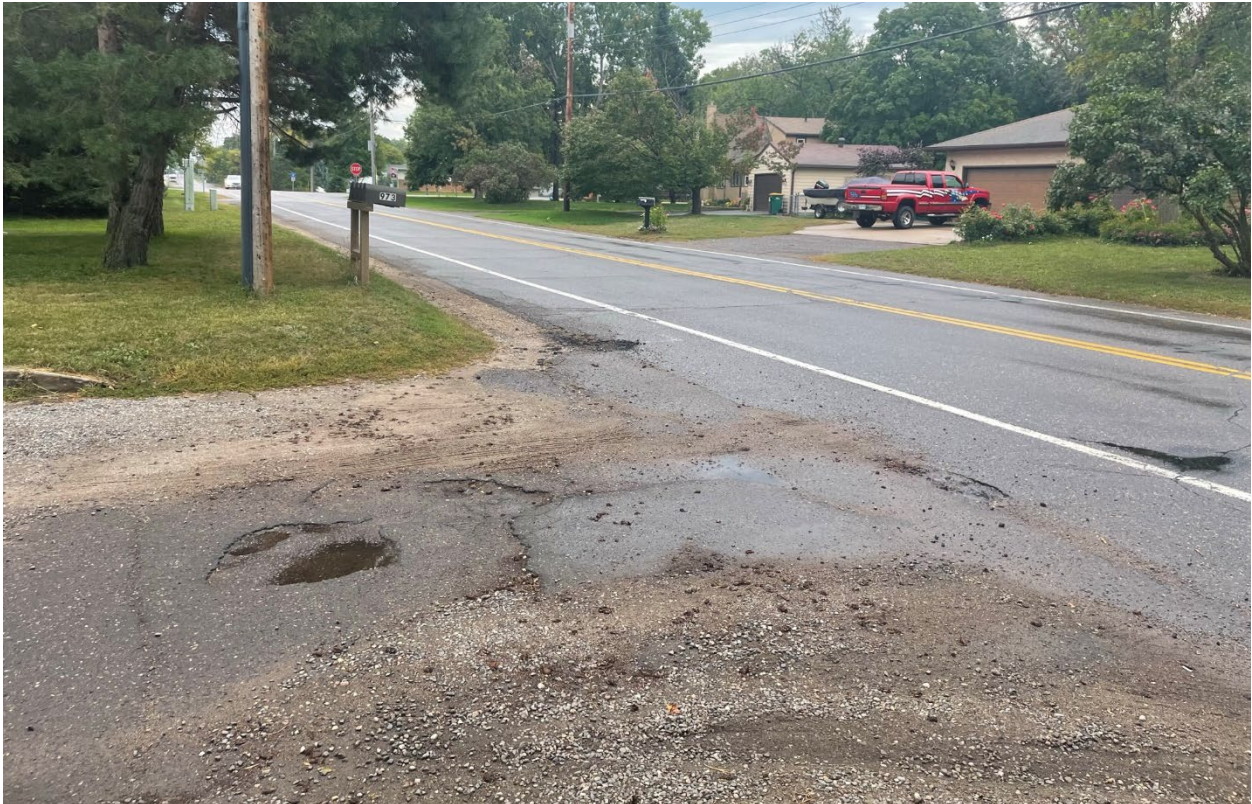
Figure 6 – Evidence of driveway condition
