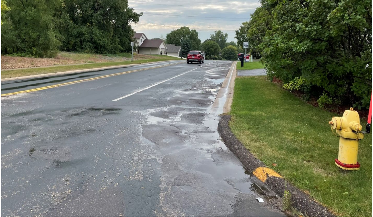
Figure 7 – Additional evidence of roadway condition
