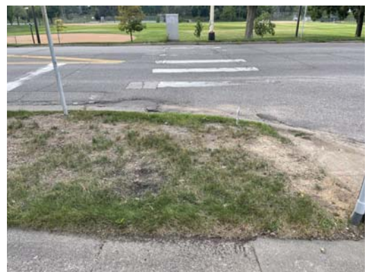
Intersection lacks ramp to align with the marked pedestrian crosswalk along Portland Ave (CSAH 35) and E 54th St.
