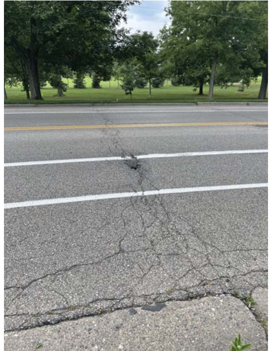
Pavement along the roadway contains cracks and requires repair similar to the image above. A mill and overlay is anticipated to be completed in coordination with this pedestrian project.
