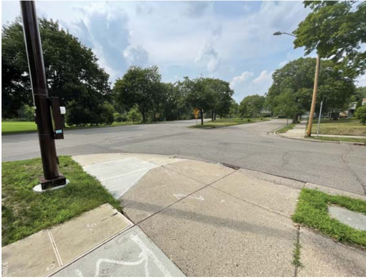
The intersection of Portland Ave (CSAH 35) and E 52nd St is pictured above. The intersection lacks ADA compliant ramps.
