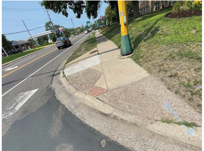
This intersection lacks ADA compliant truncated domes and sufficient ramps for people to walk and roll.
