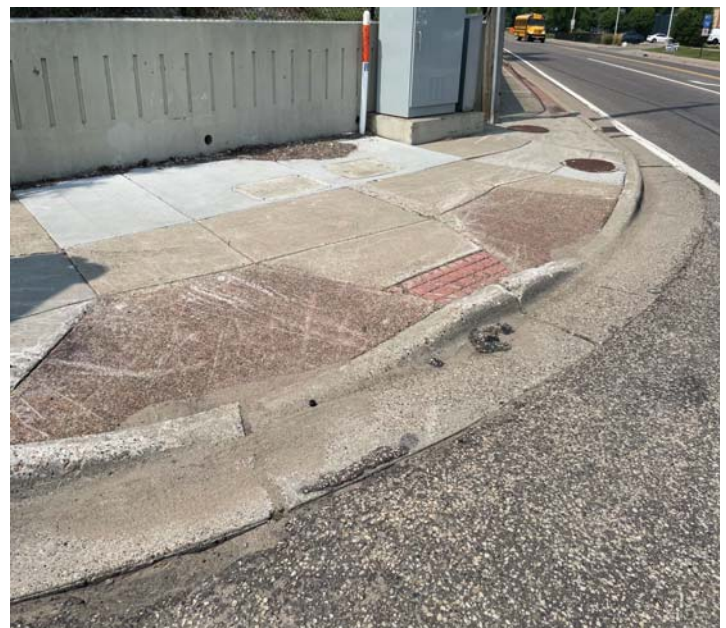
Ramps along the roadway lack truncated domes and need to be updated to current ADA standards.
