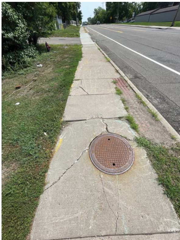
Sidewalk along roadway contains cracks and requires repair for people walking and rolling.
