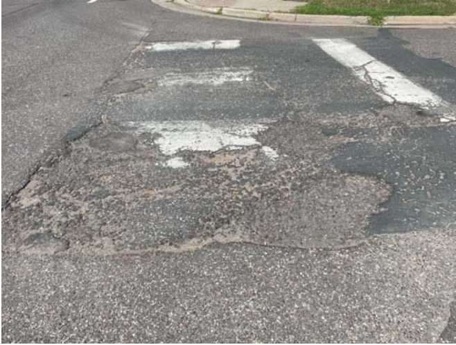
Pavement infrastructure is cracked and requires repairs. Upon completion of this project, Hennepin County plans to complete an overlay to provide a smooth surface for people driving and people biking.
