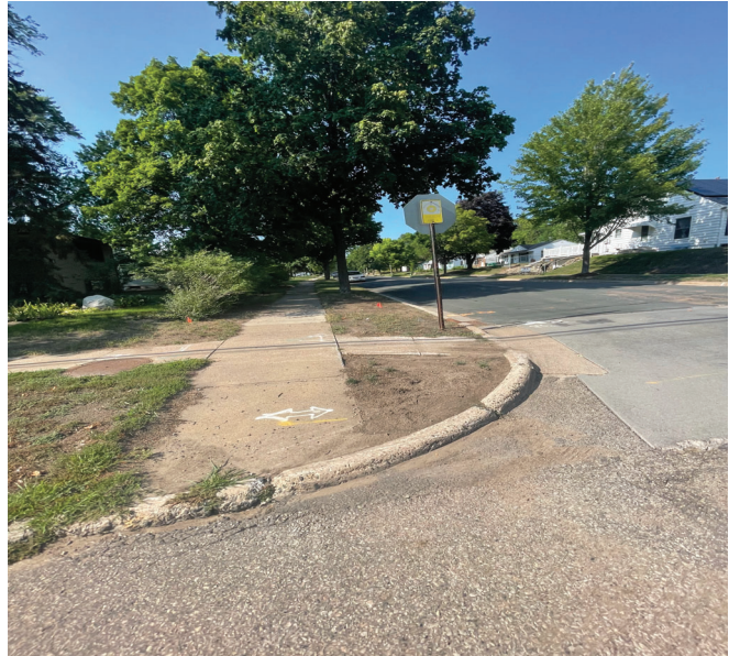
Many intersections along Minnetonka Blvd (CSAH 5) like Dakota Ave and Minnetonka Blvd (CSAH 5) lack ADA compliant pedestrian ramps.
