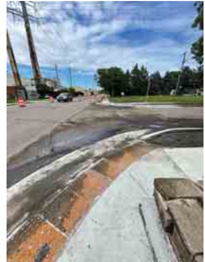
The intersection of Marshall St NE (CSAH) 23 and NE 28th Ave pictured above. Pavement prone to flooding will be addressed through this project
