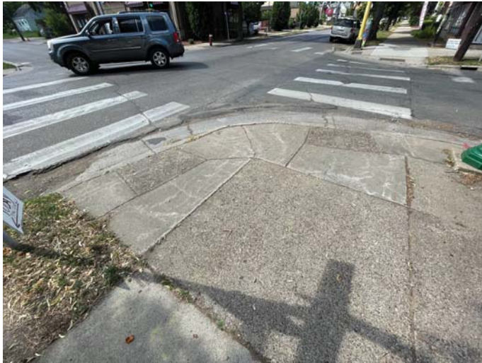
The intersection of Cedar Ave (CSAH 152) and E 34th St is pictured above. This photo shows aging pedestrian and roadway infrastructure as well as non-compliant curb ramps.
