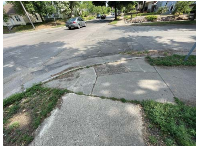
The intersection of Cedar Ave (CSAH 152) and E 45th St is pictured above. This crossing lacks ADA compliant pedestrian ramps.
