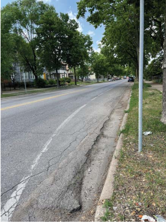
Curb and gutter along Cedar Ave (CSAH 152) is aging and requires repair.
