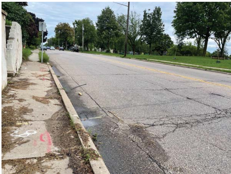
Roadway infrastructure is beyond its useful life and requires replacement.
