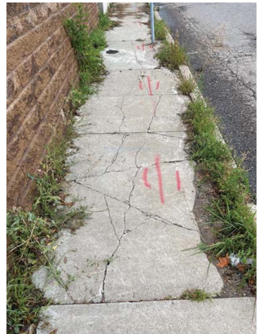
Aging sidewalk infrastructure making it difficult for people to walk and roll.
