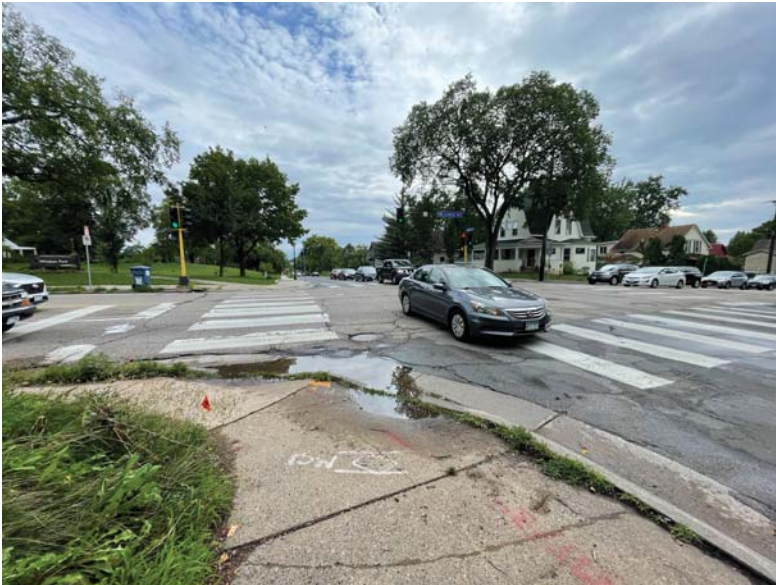
The intersection of Lowry Ave NE (CSAH 153) and Johnson St NE is pictured above. Ramps along the corridor are not ADA compliant. Insufficient storm water management along the corridor leads to flooding obstructions at intersections.
