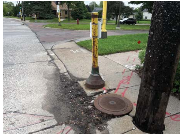
Sidewalks and pavement are aging and require replacement. There are many obstructions along the corridor for people walking as shown above at Kenzie Terr (CSAH 153) and Stinson Pkwy.
