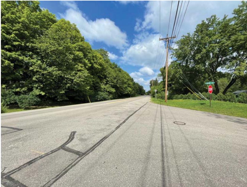
The corridor lacks consistent ADA compliant pedestrian ramps as shown in the example above in the intersection of Mill St (CSAH 82) and Brand Circle.
