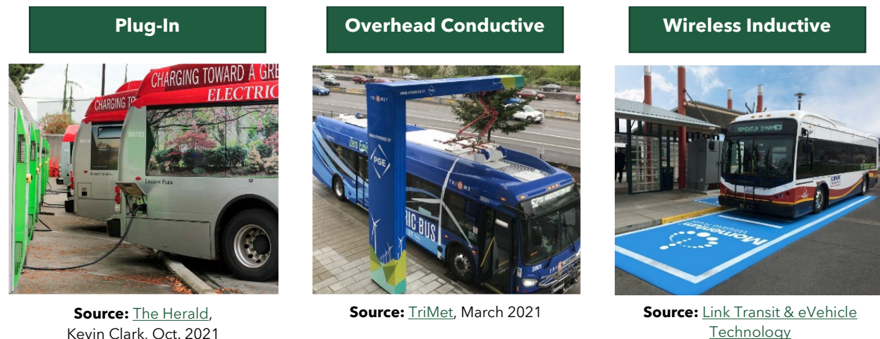
Figure 5: BEB Charging Infrastructure
