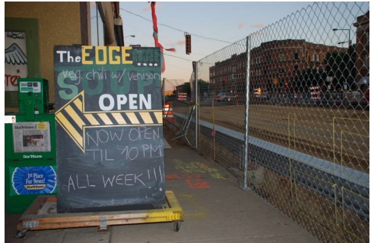
Sidewalk access is maintained behind the construction fence to the Edge Coffeehouse just west of Raymond and University
