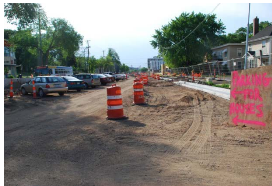
Photo 1: Contractors created temporary parking for residents in the construction zone on University Avenue in Minneapolis.
