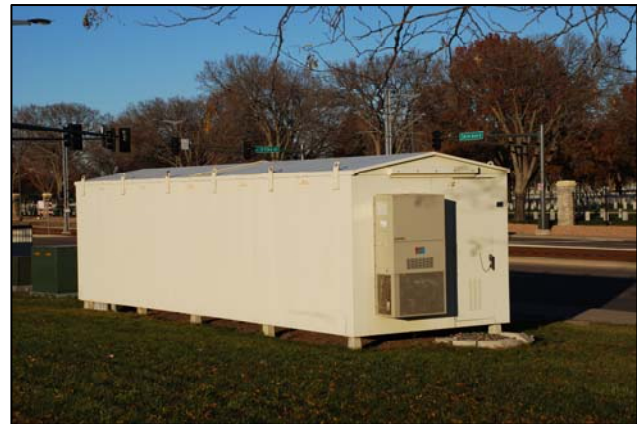
Traction power substation
