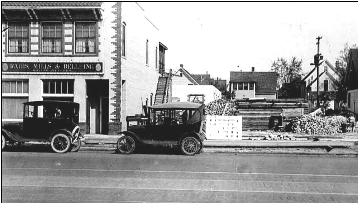
The addition to Raths, Mills and Bell, Inc. is being constructed at the rear of the site, 1921.
