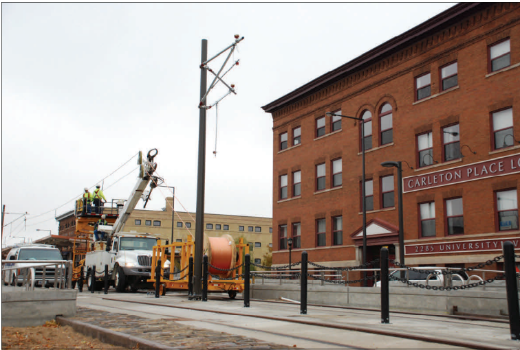
Installation of wires for overhead catenary system that will bring power to the trains near Raymond Avenue Station.
