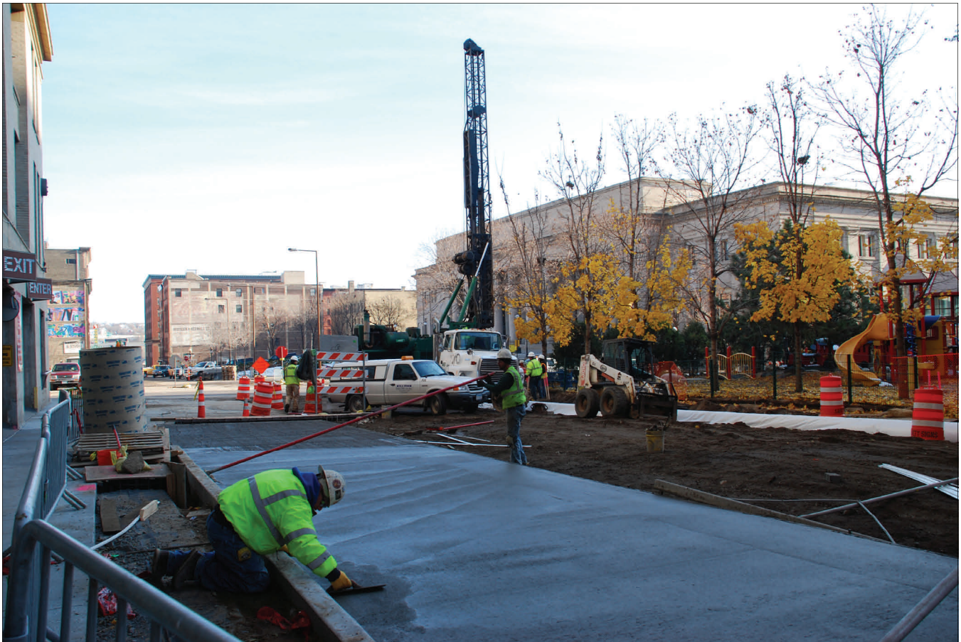
In mid-November, crews paved Fourth Street in front of the Sibley Square Ramp.
