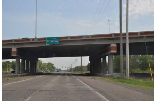
Figure 14 - View south along Bottineau Boulevard approaching the Interstate 94 overpass bridge. BNSF right of way at right.
