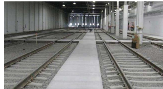
Interior storage tracks, Central Corridor OMF.
