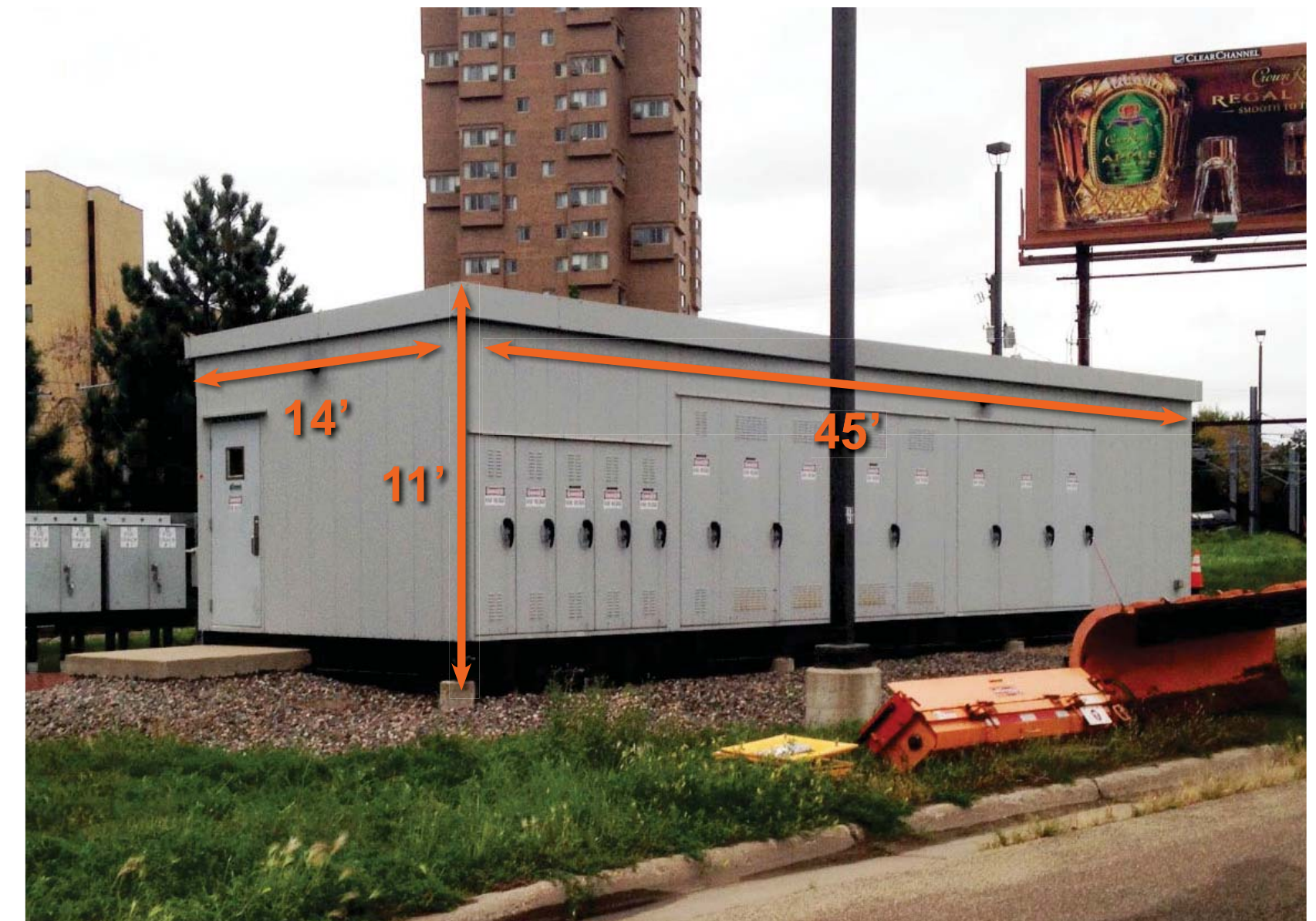
Existing TPSS along the Blue Line
