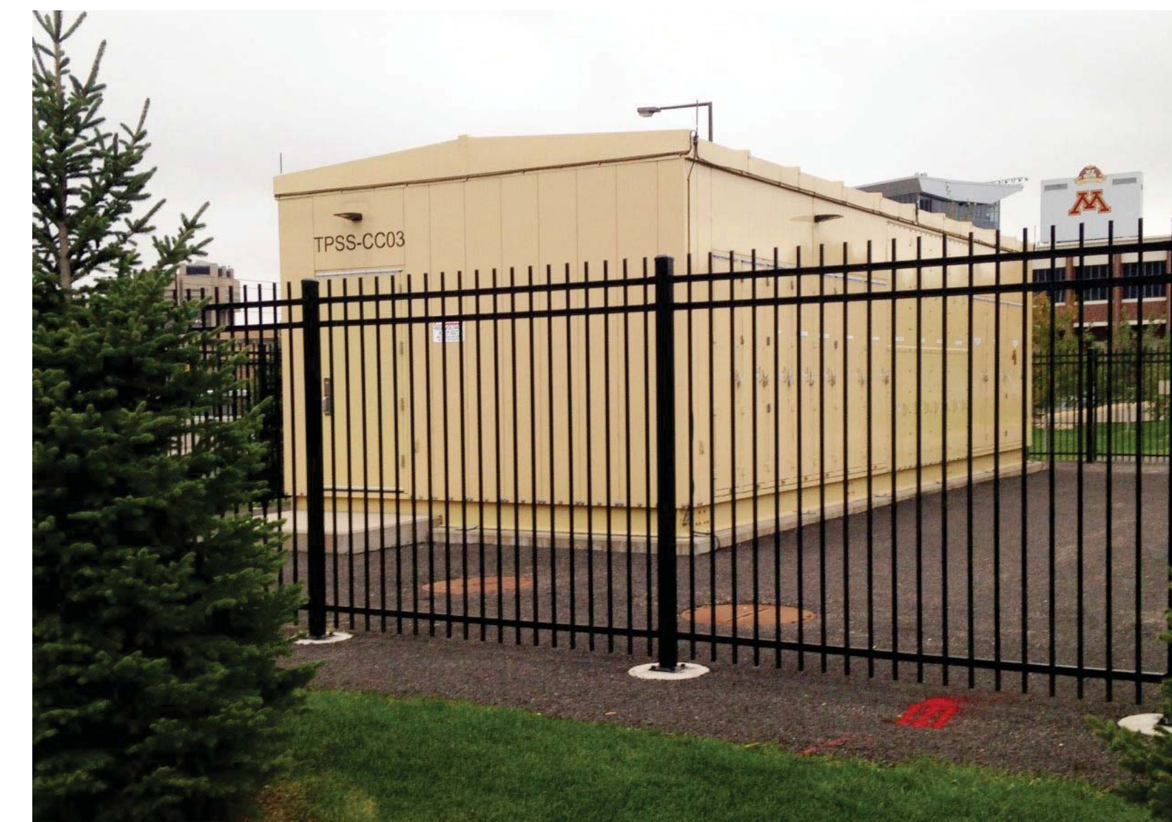
Existing TPSS along the Green Line
