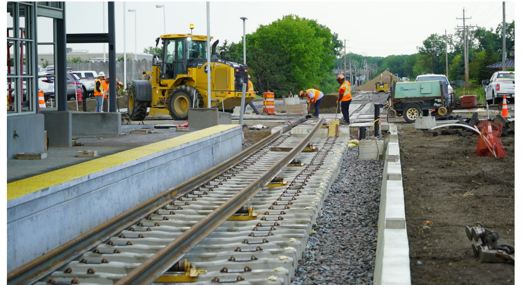
LRT track at the Downtown Hopkins Station
