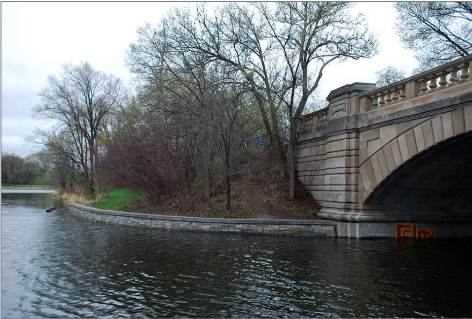
Figure 66. Classical Revival Limestone Shoreline Retaining Wall on NW side of Bridge No. 4, facing north
