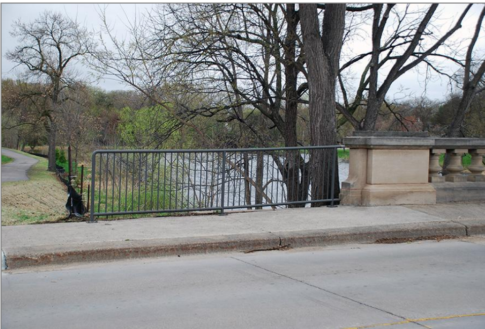
Figure 81. Tube Steel Railing located at the west side of the south end of Bridge No. 4, facing northwest
