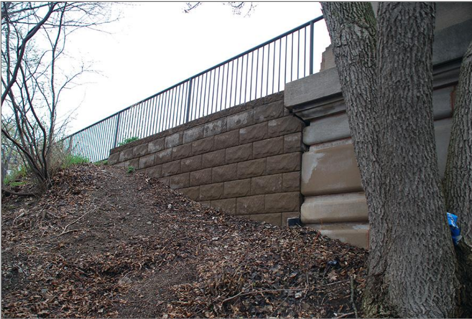
Figure 73. Concrete block retaining wall located on the east side of the south end of Bridge No. 4, facing southwest
