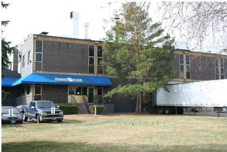
Figure 75. Northeast corner of Building #1, the prestressed concrete panels were added as part of the 1968 building addition, view facing southwest.
