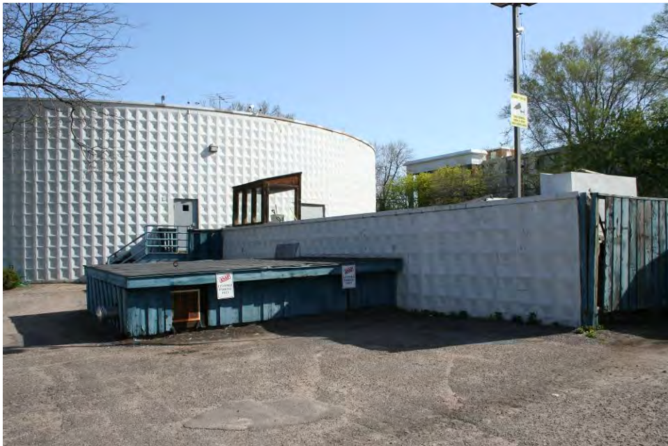
Figure 83. Loading dock on the south portion of the building, view facing southeast.
