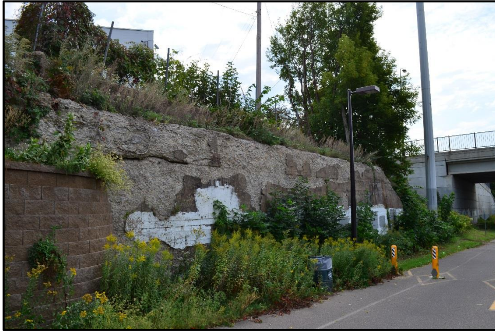
Figure 23. Modern concrete block wall (left) and deteriorated historic formed concrete retaining wall with secondary wall above (right) on the east/southeast side of the corridor north of 12th Street, August 2017
