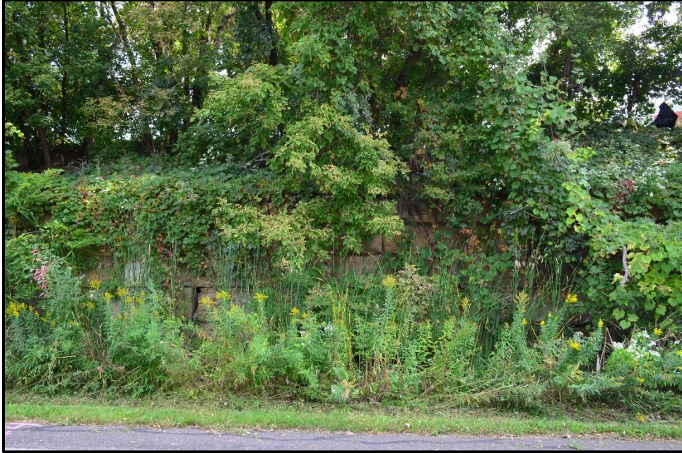
Figure 25. Historic stone masonry retaining wall east of Glenwood on east/southeast side of corridor, August 2017
