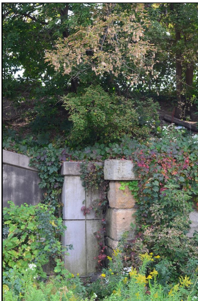
Figure 24. End of 12th Street Bridge abutment and beginning of historic stone masonry retaining wall extending to Glenwood on east/southeast side of corridor, August 2017
