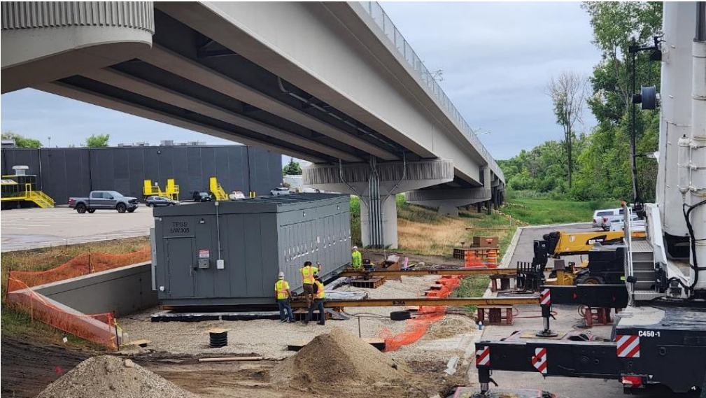
TPSS SW305 Installation in Eden Prairie
