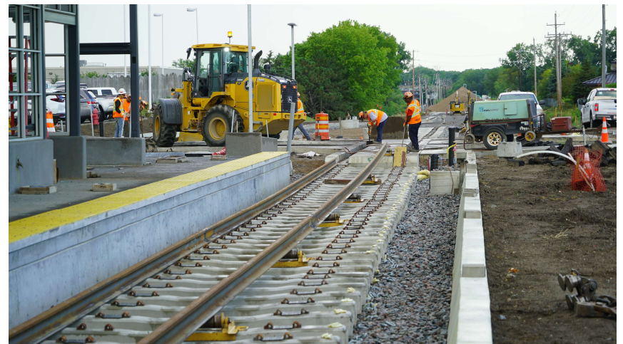
LRT track at the Downtown Hopkins Station
