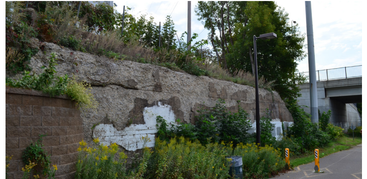
Remnants of a historic masonry retaining wall in the corridor protection area
