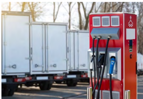
Figure: An electric truck charging station
