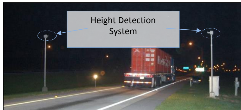
Figure 4-33. Height Detectors on Weigh Station Ramp
