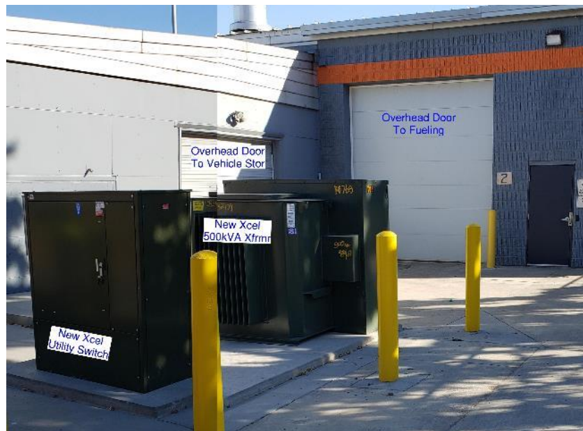
Figure 45 - Transformer & Utility Switch
