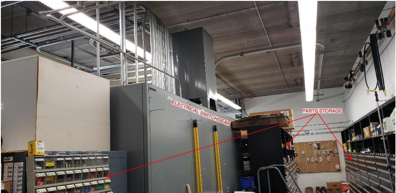
Figure 53 - Existing Switchgear Land Locked in Parts Room
