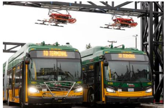
Figure 33. King County Metro Gantry Charging System
