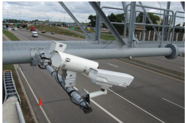
Figure 30: Enforcement Assistance CCTV Camera
