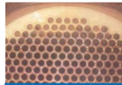
Auxiliary Condenser Improvements
