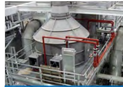
Wet ESP Improvements
