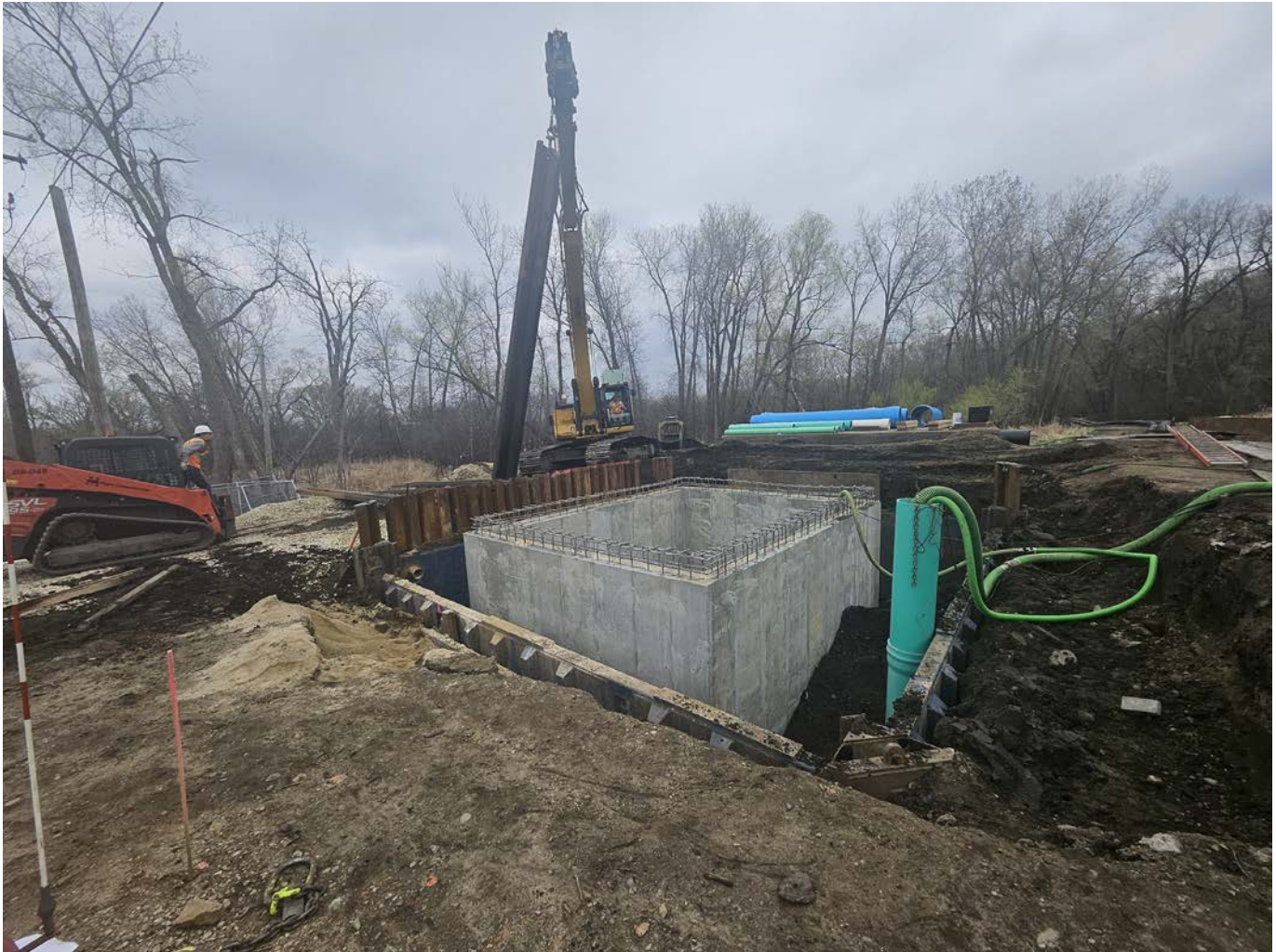
The construction of a new outfall structure for the Bloomington siphon in Eagan
