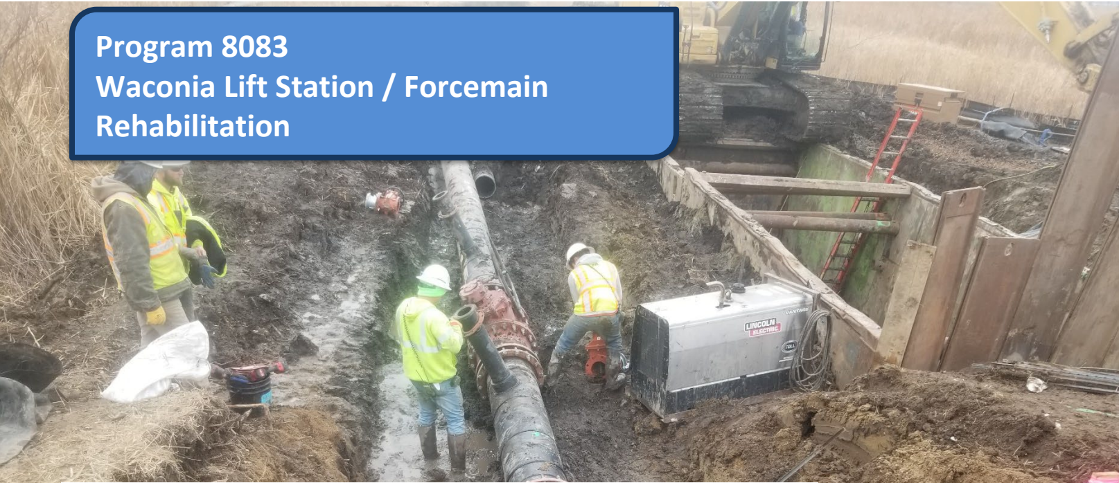
Contractor installing interim conveyance near the micro-tunnel pit on the west side of Carver County Highway 92
