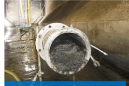
Sludge Storage Mixing Improvements
