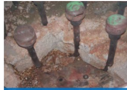
Fluid Bed Incinerator Air Distribution
