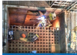
Baghouse Stainless Steel Liner
