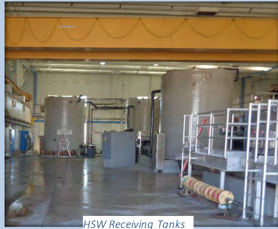
HSW Receiving Tanks
