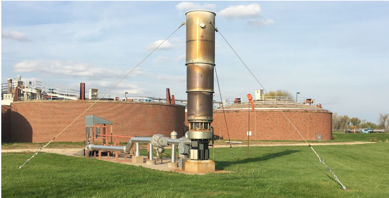
Biogas flare and Digesters 4 and 5 at Empire WWTP
