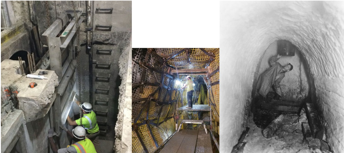
Photo collage including 4 th Street tunnel repairs and the inside of a tunnel constructed in the 1930s.
