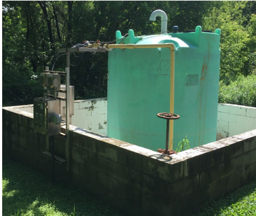
L-24 Chemical Odor Control Tank and Pumping System
