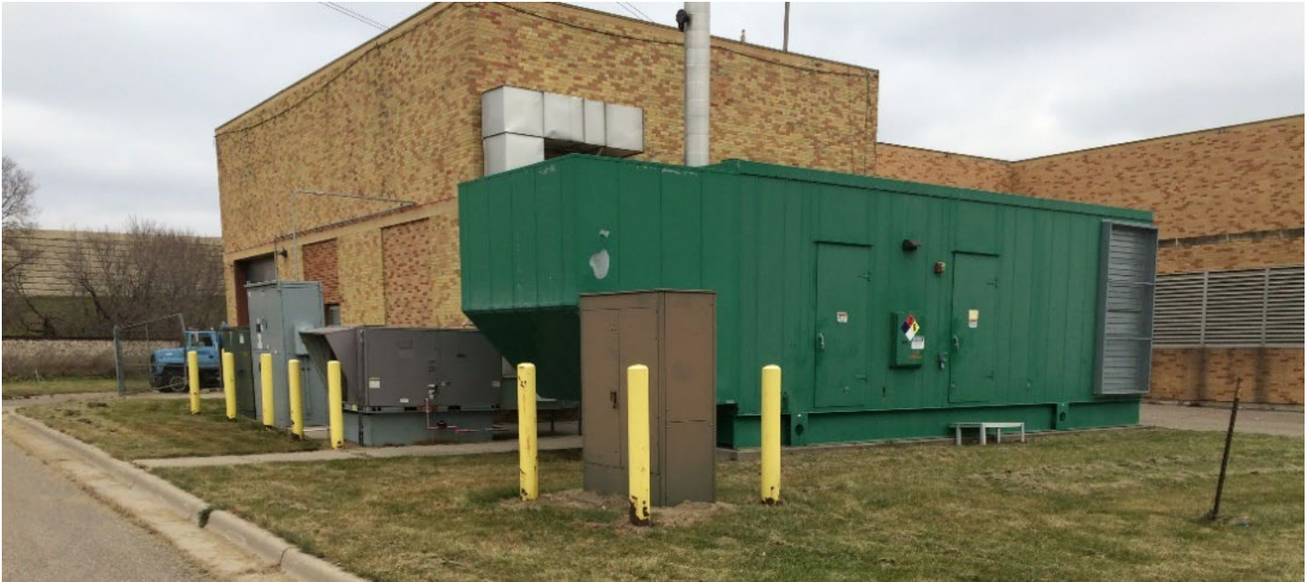
Backup generator at Metro WWTP
