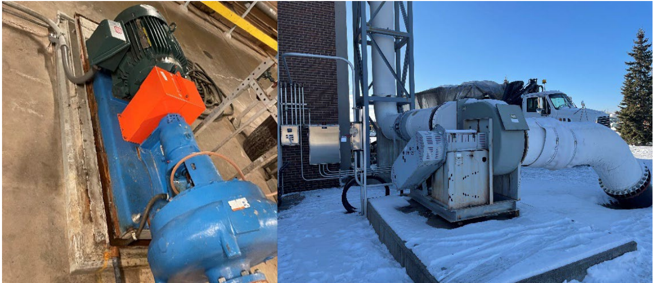
Left: Primary sludge pumps. Right: Odor control fan
