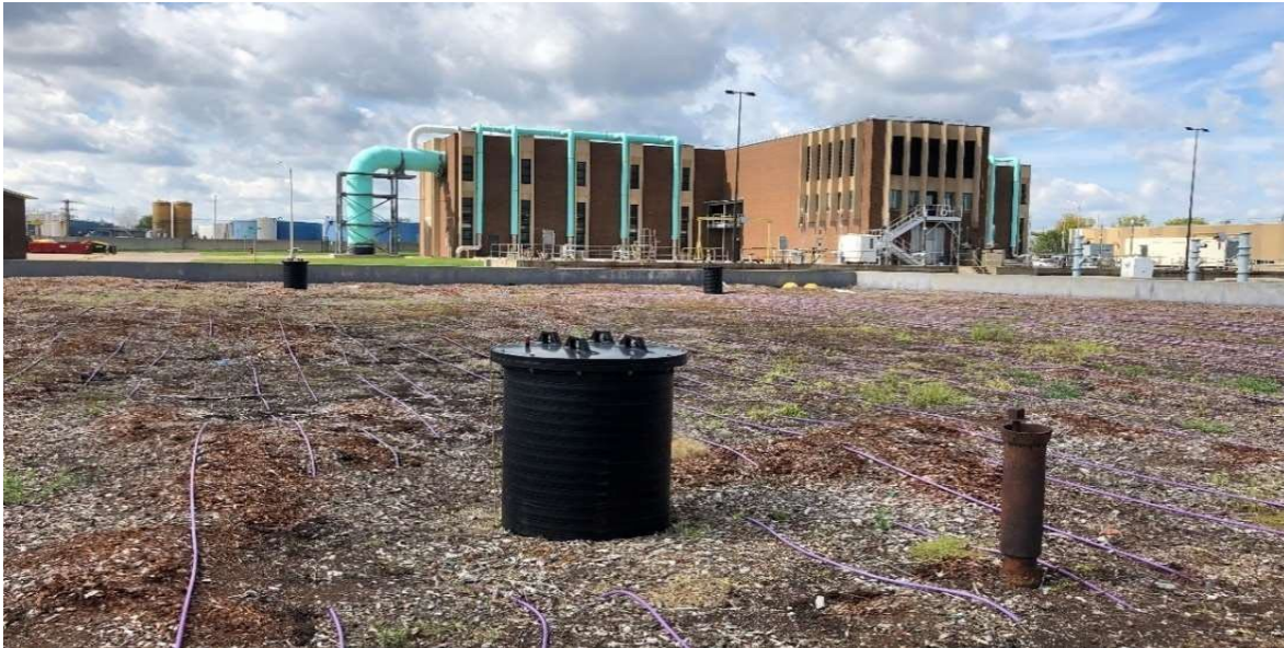
Existing East Pretreatment Biofilter
