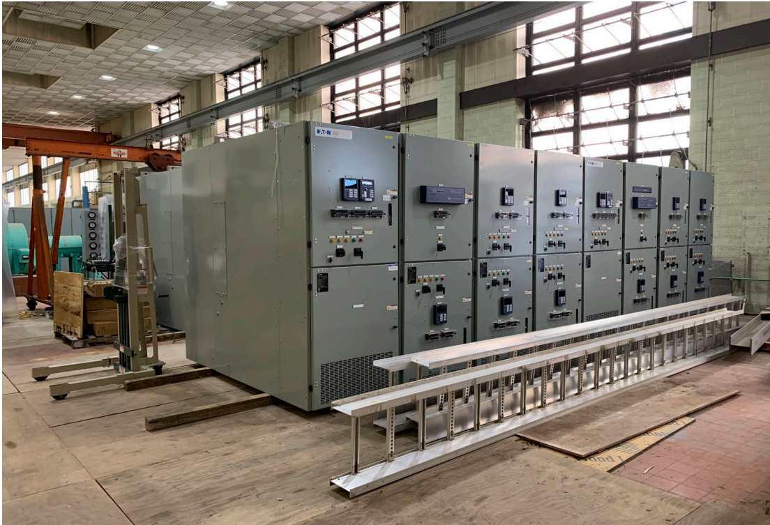
New unit substations to be installed
