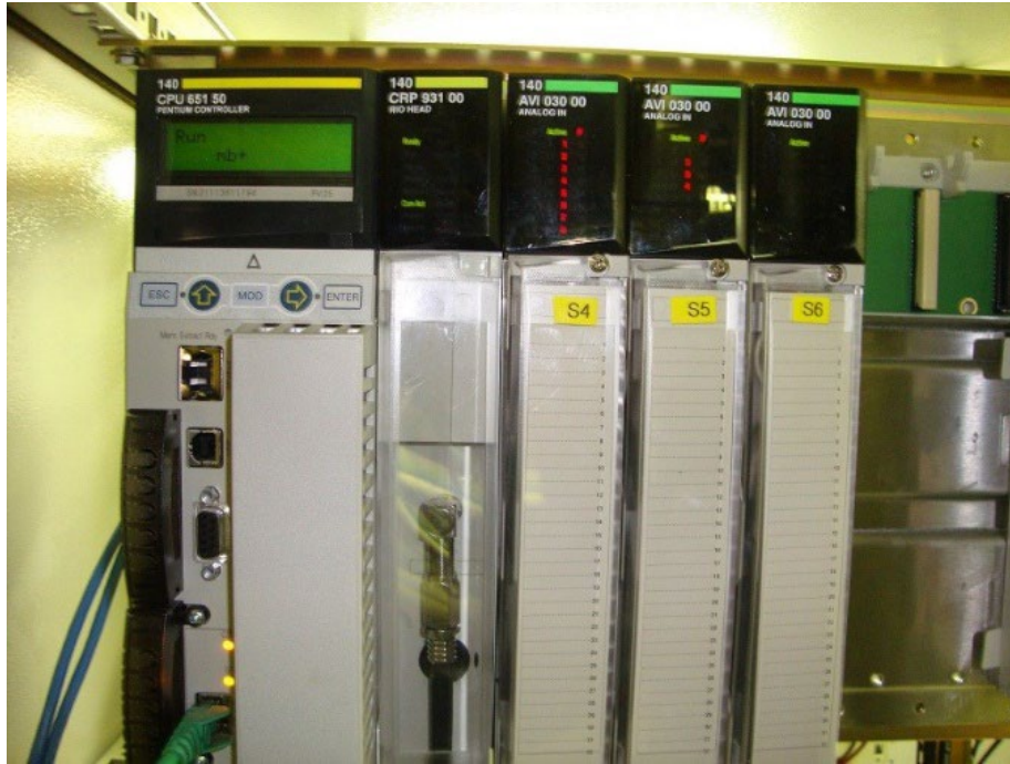
Typical PLC (Programmable Logic Controller)
