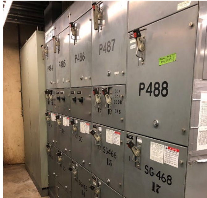
Motor control center
