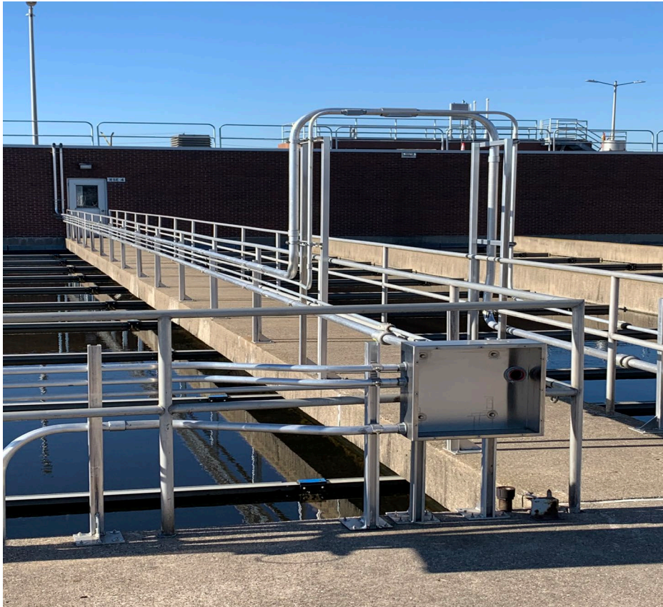
Electrical Conduit for Secondary Collector Motors
