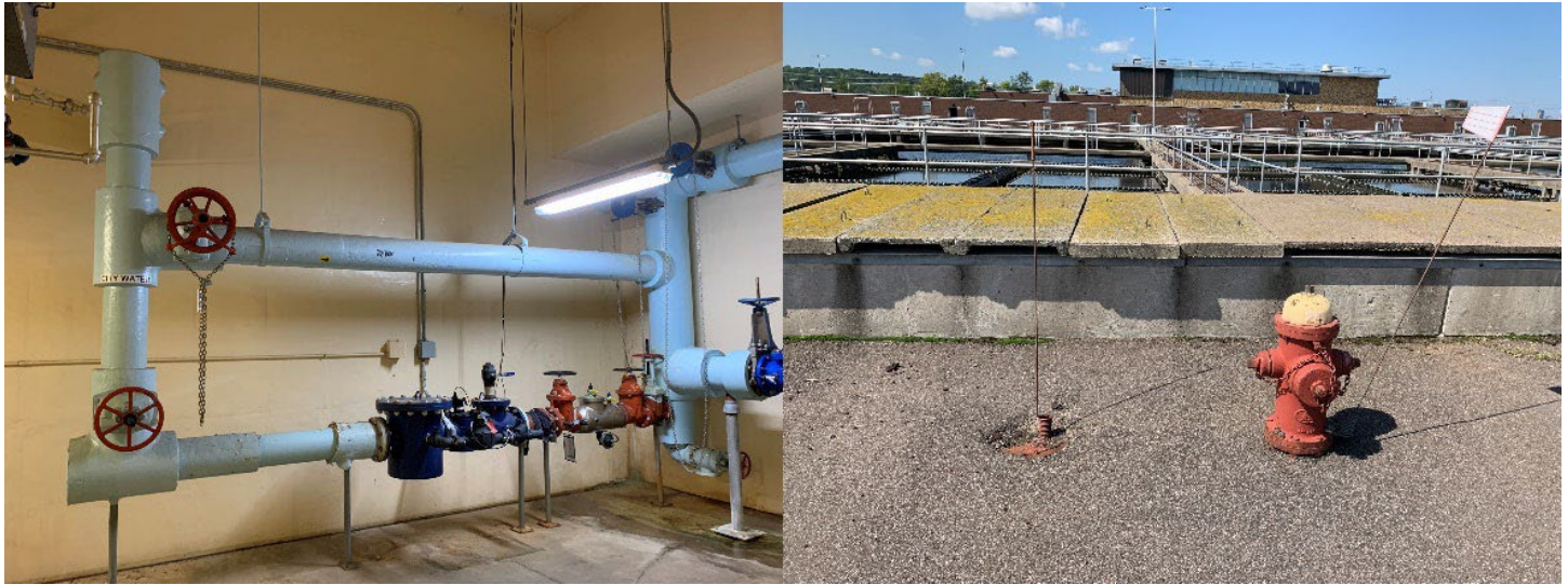
Left: One of two water metering stations which is located near East Primary. Right: City water hydrant and isolation valve at final sedimentation tanks.
