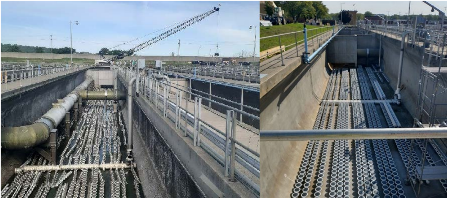
Left: Demolition of diffusers - Metro Plant's secondary treatment. Right: Installation of diffusers - Metro Plant's secondary treatment.
