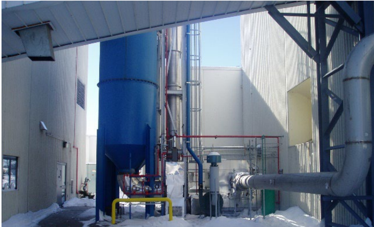
Existing Regenerative Thermal Oxidizer
