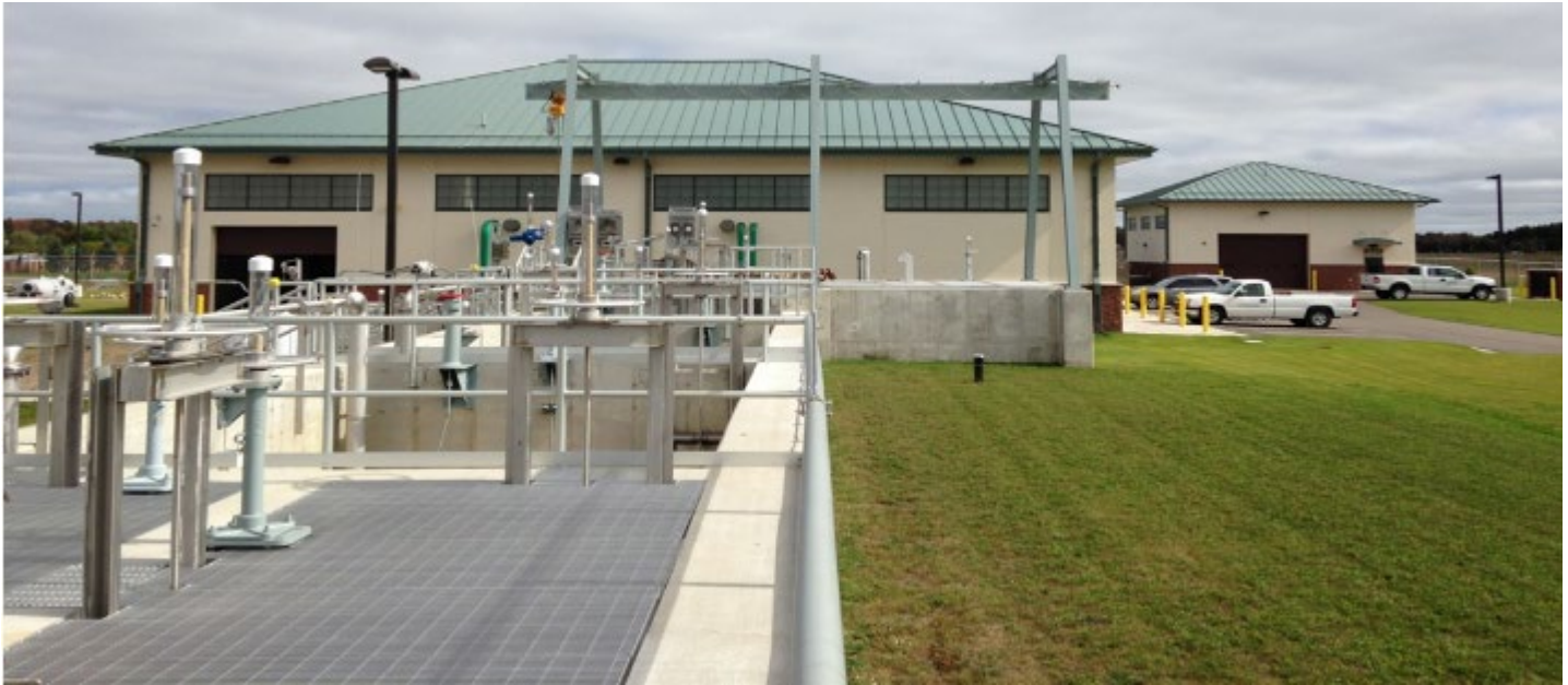
East Bethel Water Reclamation Plant
