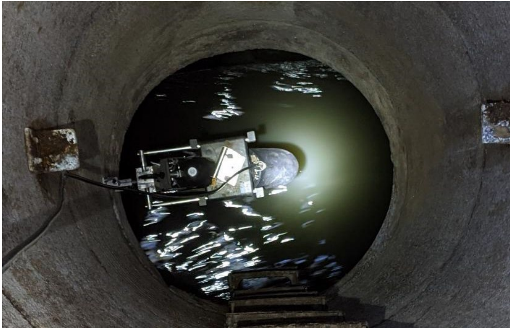
Photo of a LaserFlow flow monitor inside ES interceptor pipe
