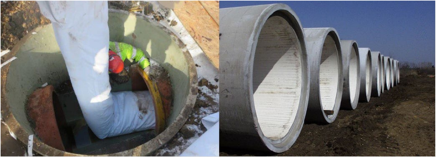
Left: Cured-in-Place (CIP) pipe liner being installed through a maintenance hole. Right: Large-diameter interceptor sewer pipe segments ready for installation.
