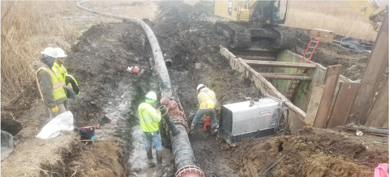
Contractor installing interim conveyance near the micro-tunnel pit on the west side of Highway 92 in Carver County
