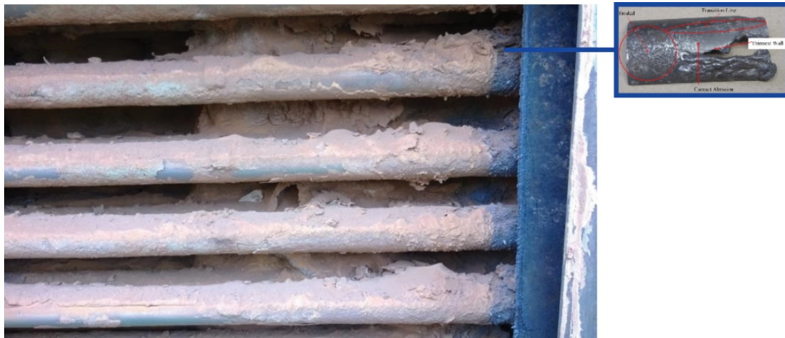
Photo 4. Forensic examination determined that abrasion between the tube and the tube sheet had caused failures in this area (economizer, incinerator train 2).
