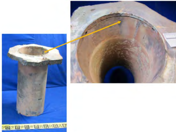
Photo 3. Cracking in the primary heat exchanger tubes at the tube sheet will cause the tubes to fall out of the tube sheet.
