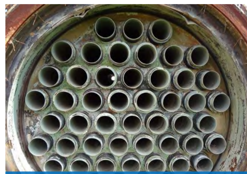
Primary Heat Exchangers
