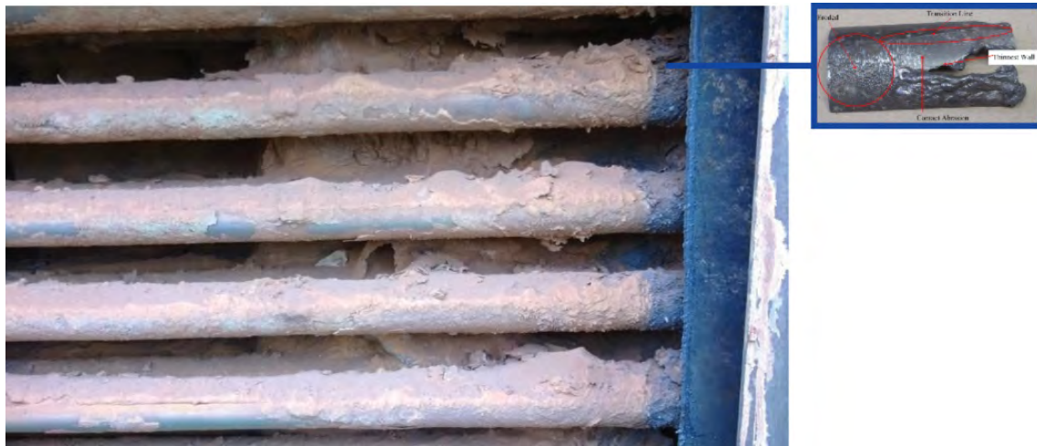
Photo 4. Forensic examination determined that abrasion between the tube and the tube sheet had caused failures in this area (economizer, incinerator train 2).
