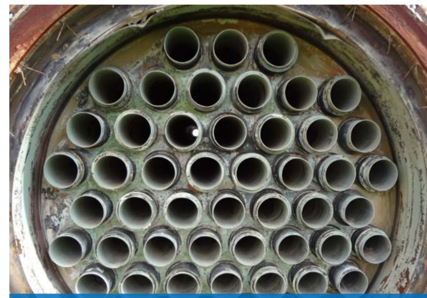
Primary Heat Exchangers
