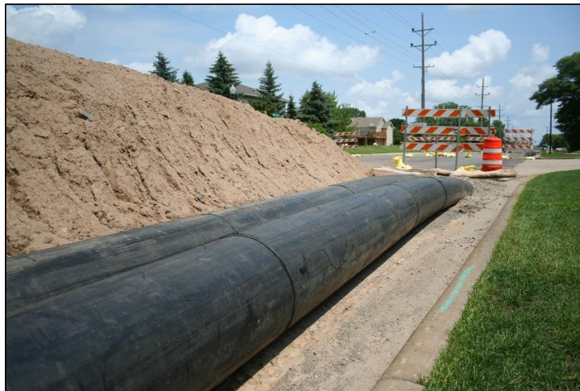
MCES crews bury temporary wastewater conveyance pipes at intersections to maintain traffic access during sewer work
