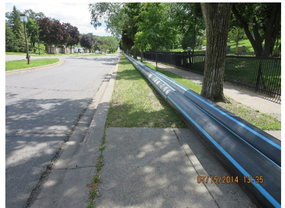
Example of above-ground temporary wastewater conveyance pipes.
