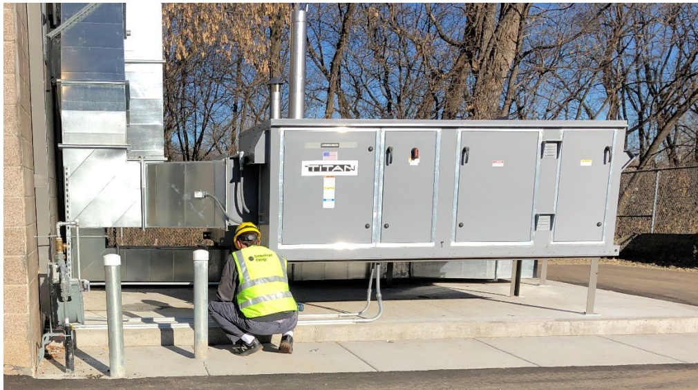
Crews are installing the new HVAC system at the lift station in Maple Plain
